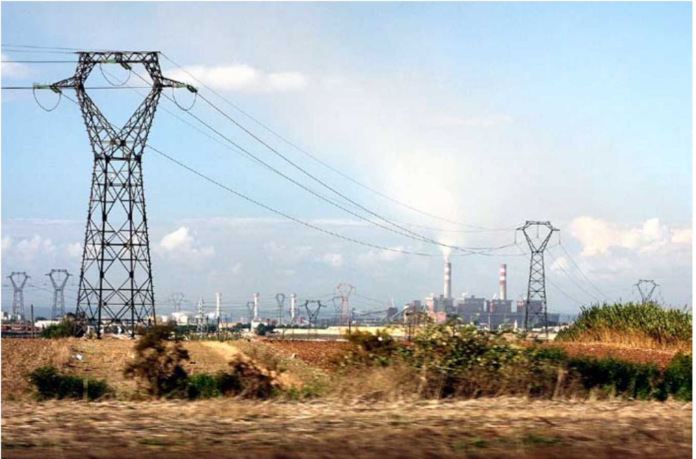
Transmission lines, Morocco (© Regina Charyparová)
