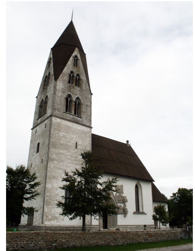
Plaster in high towers is very expensive to repair. It is necessary to periodically thoroughly examine the condition of the plaster. The Stånga church, Gotland, Sweden. Photo: Joakim Hansson.
