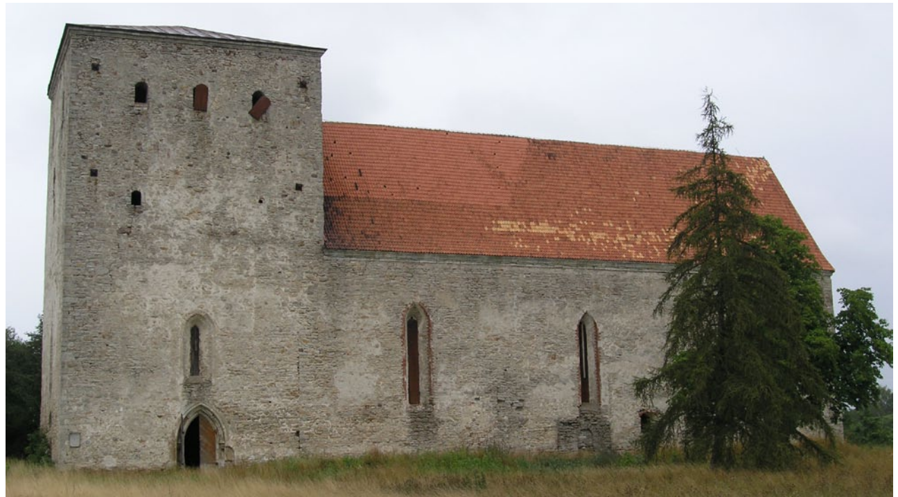
A lack of regular maintenance will lead to massive conservation work. The Pöide church, Estonia. Photo: Kaire Tooming.
