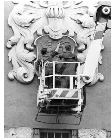
The restoration of the Tallinn coat of arms on the Estonian Drama Theatre. Tallinn's oldest symbol had been plastered over due to its similarity to the coat of arms of the Republic of Estonia.
