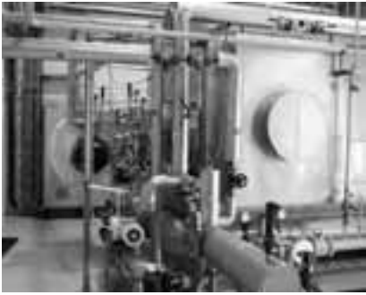
Rasvapressid, -tank ja vahemahutid. Adipose removal presses, vessel and surge tanks
