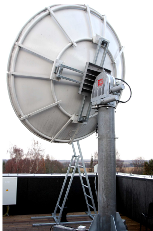
Antenna on the roof of main building. Antenn peahoone katusel.
