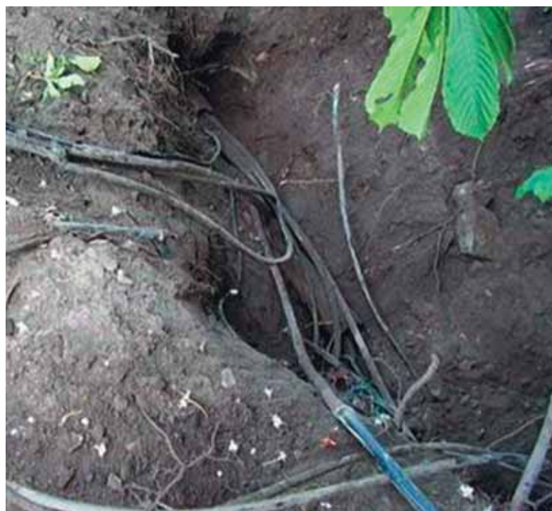
Communications cables damaged during the excavation works
