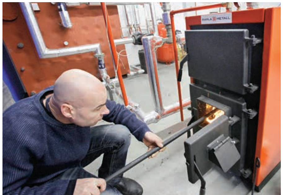
EMÜ energeetikaosakonna õppehoone uus katel, millele teeb tuld alla lektor Mart Hovi. The new boiler in the Energy Studies Building of the Estonian University of Life Sciences, lit by lecturer Mr Mart Hovi.
