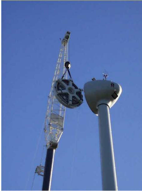
Joonis 1. Tuuliku generaatori montaaž Virtsus Figure 1. Installation of the generator to the wind-turbine in Virtsu
